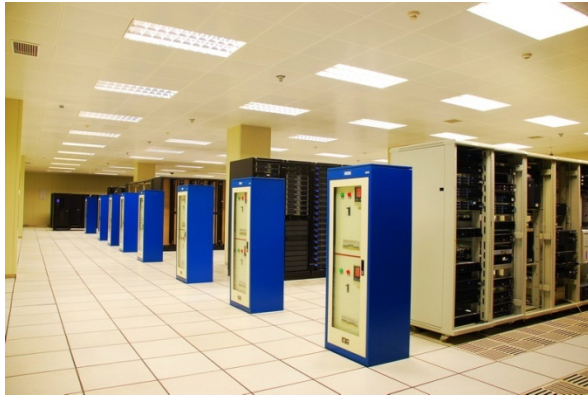
Power supply, cooling
