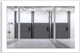
Computer Room Air Conditioner
