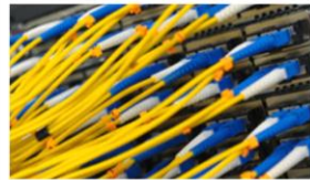
Fibre Optic & Data Structured Cabling System
